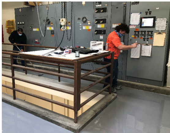
Above: Crews are working on coating the floors inside the lift station
