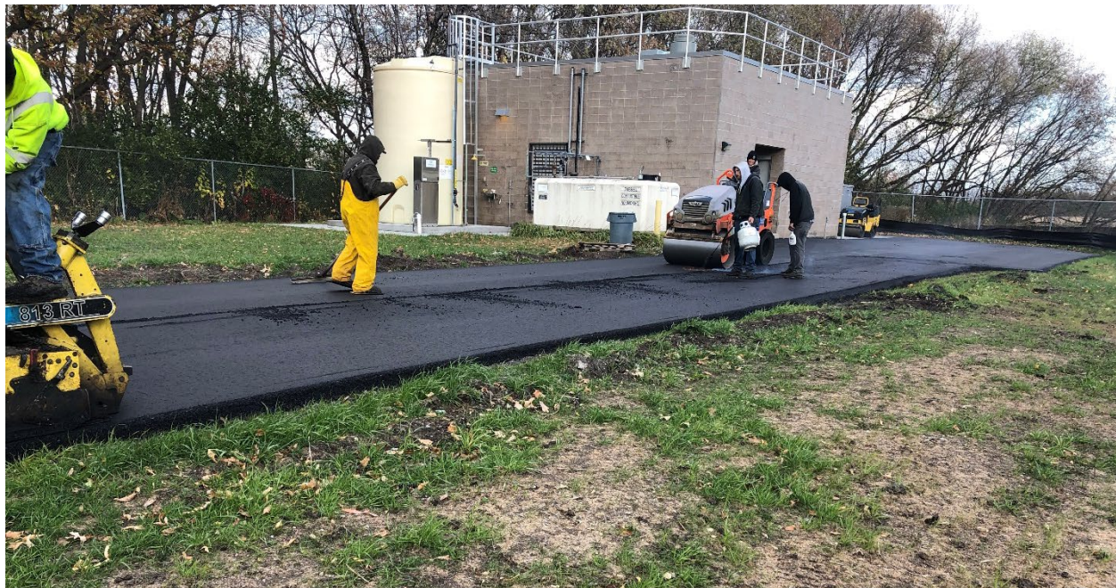
Crews are paving the new asphalt driveway at the MCES lift station in Maple Plain
