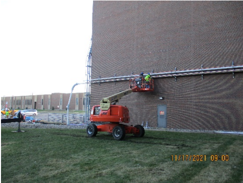
Lime and Ash Conveyance Piping outside the 408 Building.
