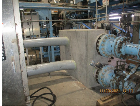
New Cake Pump Piping at SMB
