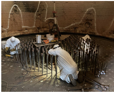
FBI3 Air Distribution Renewal
