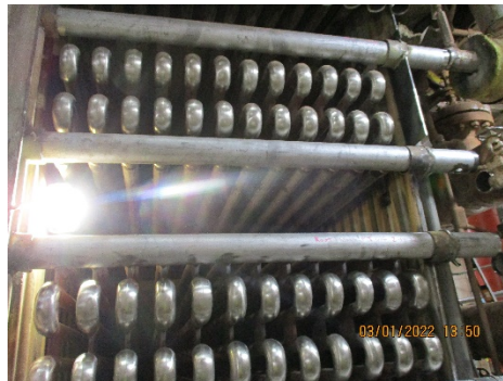
Waste Heat Boiler No. 1 New Primary and Secondary Superheaters
