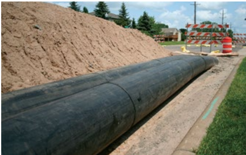
Example of above-ground temporary wastewater conveyance pipes. ►
