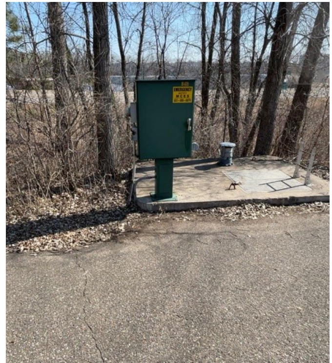
New meter structure installed near the St. Croix Trail
