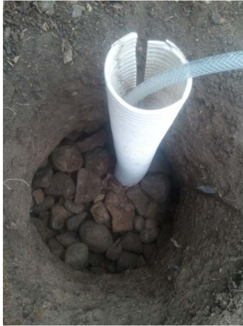
Figure A.1. Backfilling the hole during installation of the SPE20 sampler (white PVC used to protect the device during backfilling rocks at the Hamline-Midway site).
