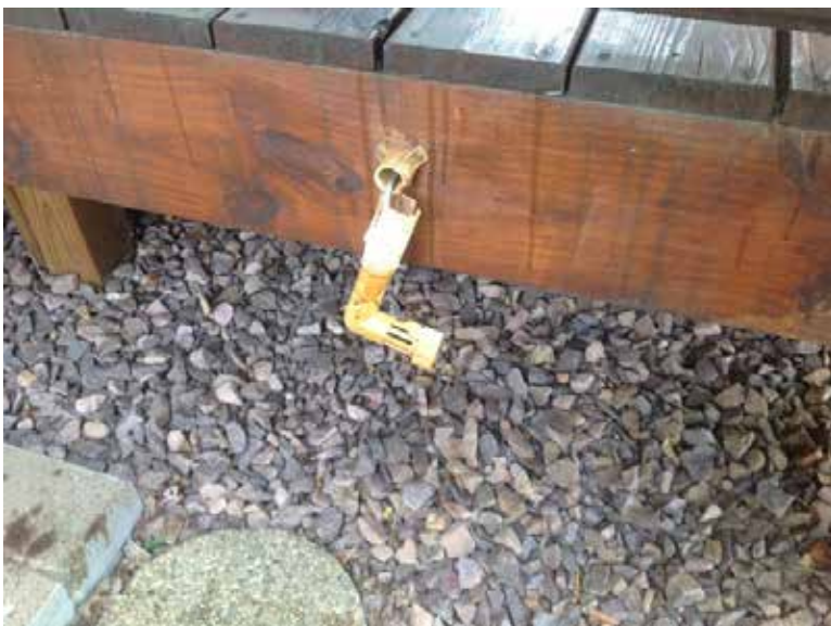
Figure 40: Example of a broken and non-functional rain sensor
