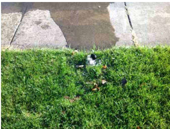
Figure 30: Example of leaking rotor head
