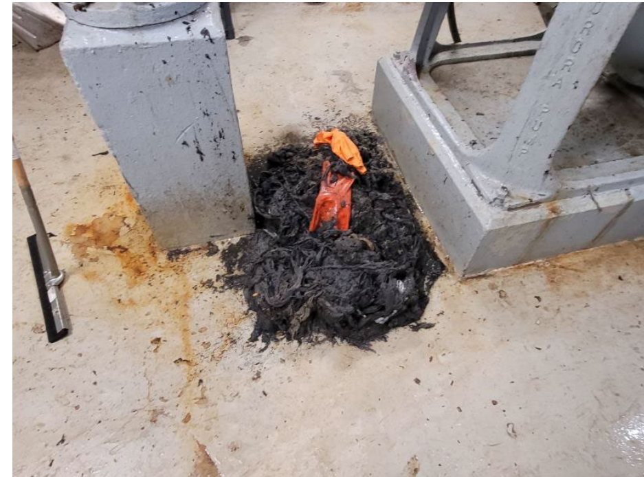
Rags removed from check valve
