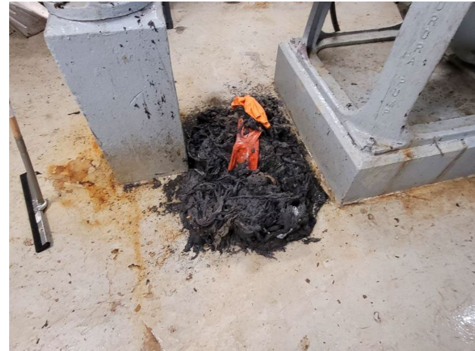
Rags removed from check valve
