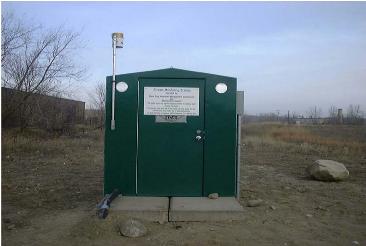
Figure WI-1: Willow Creek Monitoring Station
