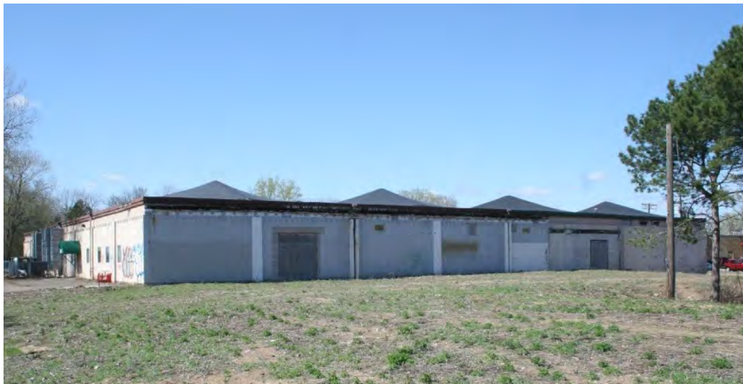
Figure 48. Northeast (side) and southeast (rear) elevations of the warehouse showing pyramidal roof structure, view facing northwest.
