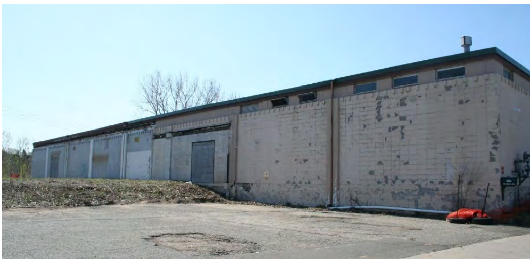
Figure 41. Northeast (side) elevation of the warehouse showing the original wall and docking bay, downspout, and foundation, view facing south.
