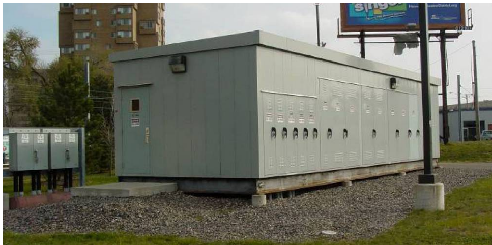
Photo 2.3-1. Typical TPSS Facility
