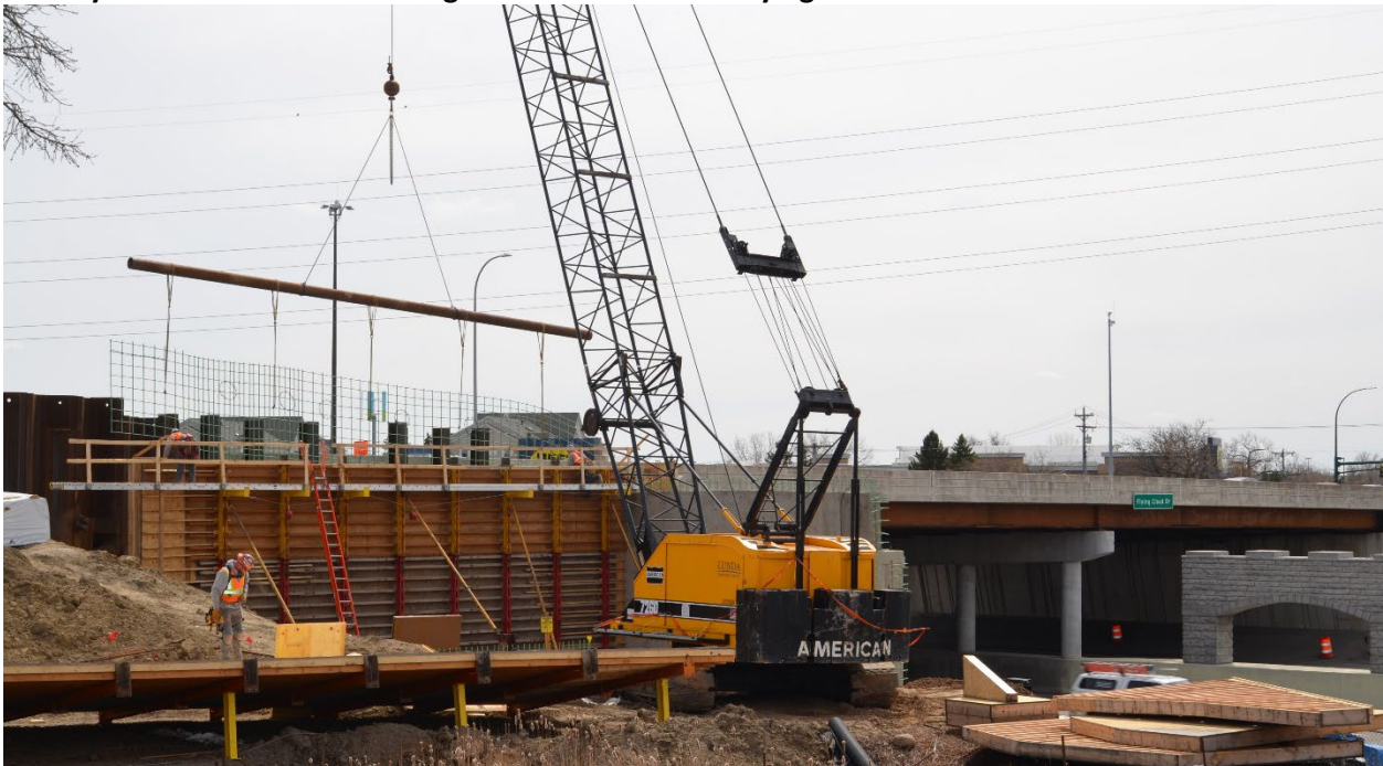
Crews work on constructing temporary forms for concrete on the approach to the bridge abutment.
