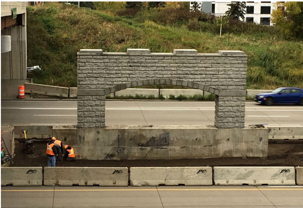
Crews work in the I-494 median to build the center pier for the LRT bridge.
