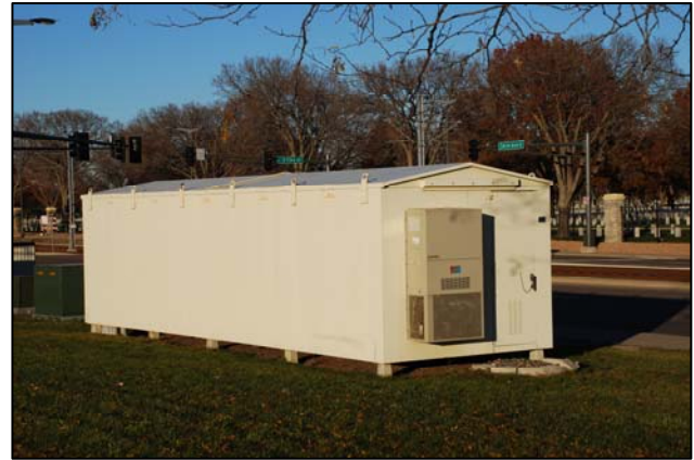
Traction power substation
