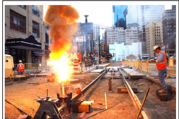
A chemical reaction turns steel rails to molten metal during the welding process. Jose Figueroa, general superintendent of rail construction for Balfour Beatty Rail, monitors the weld.
