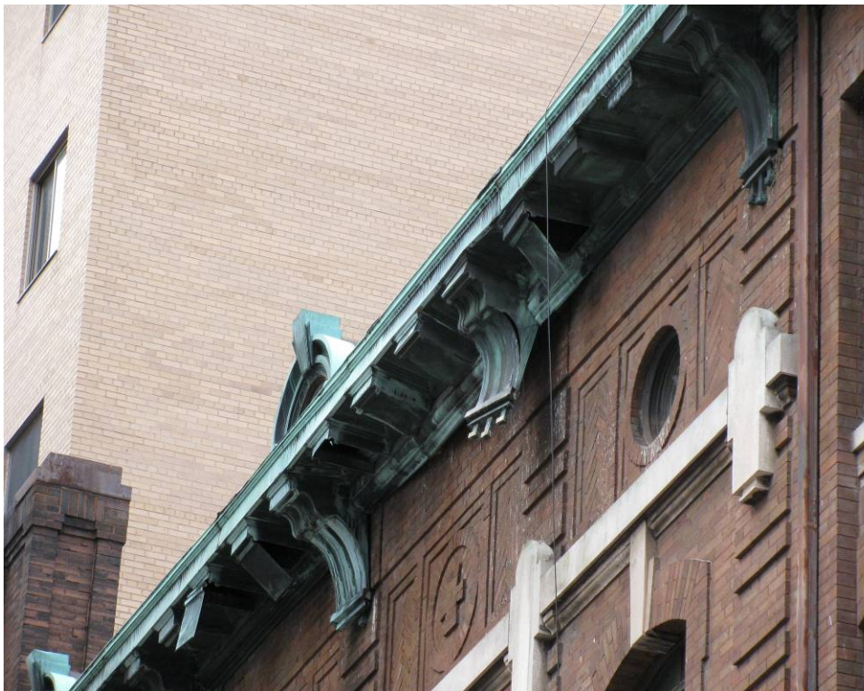
Figure 12: Loose sheet-metal on St. Agatha's Conservatory of Music and Fine Arts building
