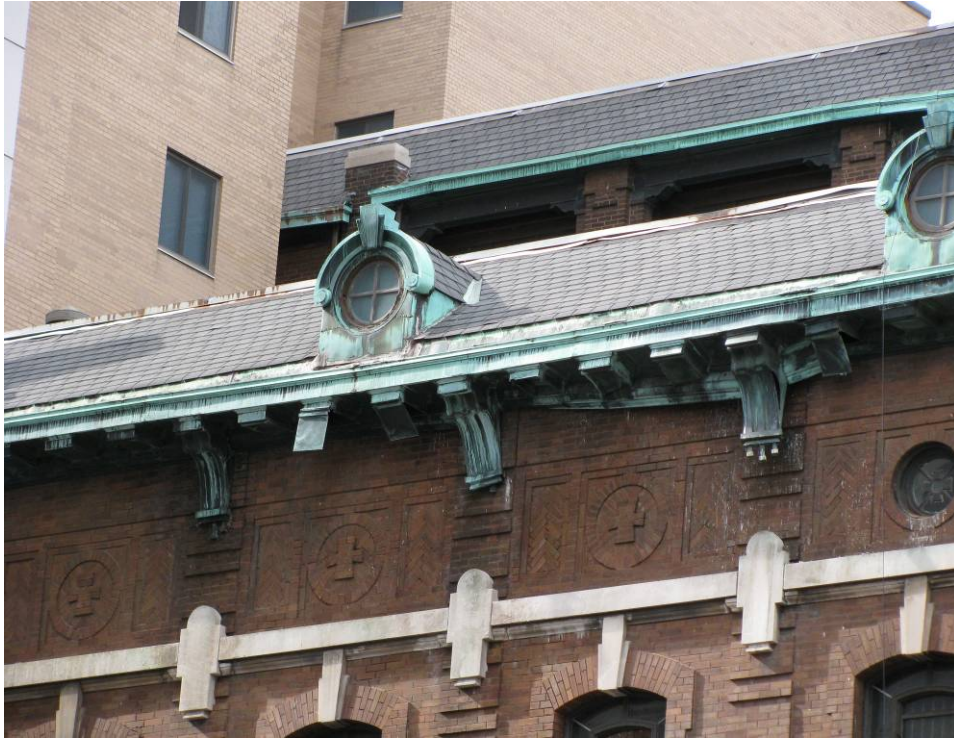
Figure 11: Loose sheet-metal on the St. Agatha's Conservatory of Music and Fine Arts building
