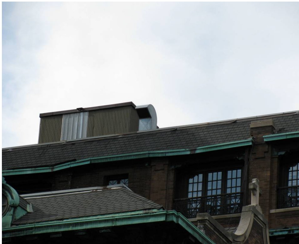
Figure 10: Loose sheet-metal on St. Agatha's Conservatory of Music and Fine Arts building
