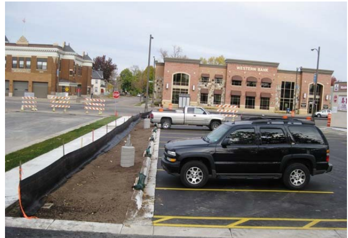
Parking lot improvements near completion at the SE corner of St. Albans and University
