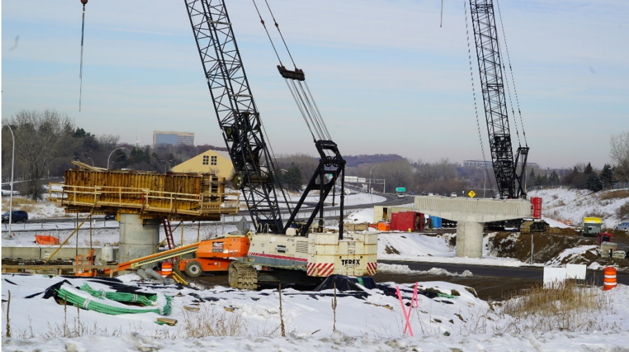
Crews are constructing multiple piers for the new LRT bridge. The various piers are at different stages of completion, with crews working on pile supports and formwork.
