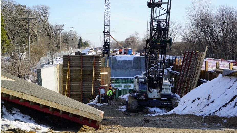
Crews work on abutments and retaining walls at Minnehaha Creek in St. Louis Park.
