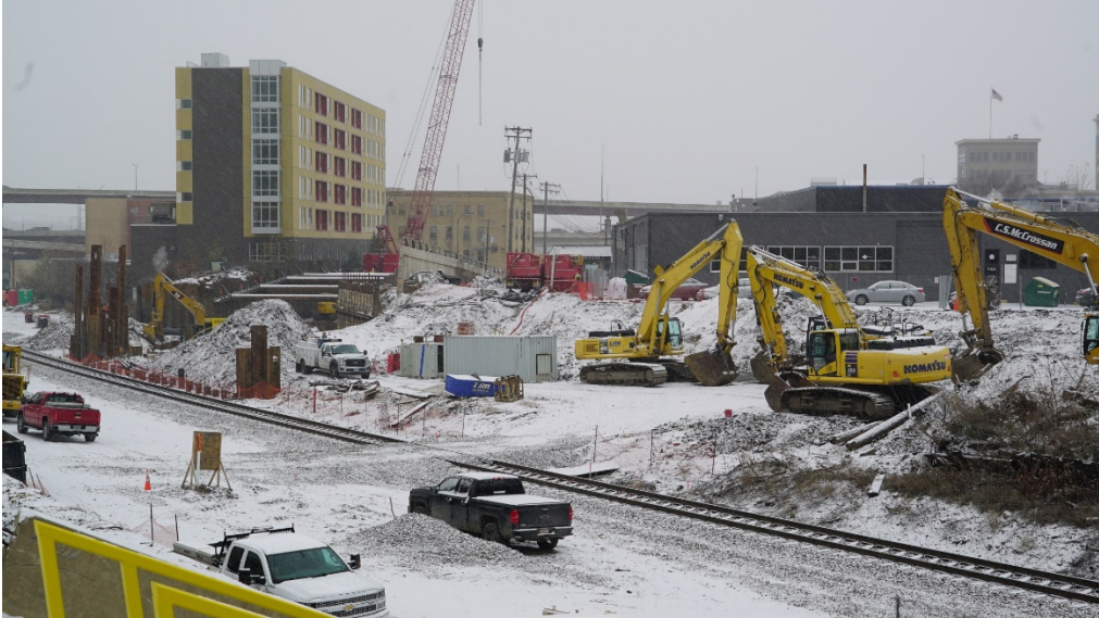
December 2019 Crews move utilities, install retaining walls, and prep for the construction of the new Glenwood Bridge.
