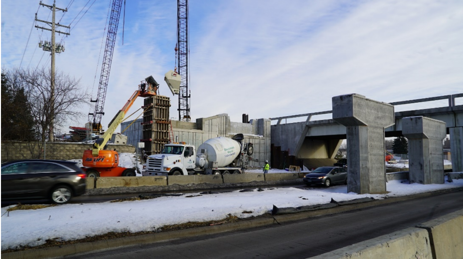
Bridge abutment and retaining wall construction is concluding and the crane, pictured, will be moving to another area of the project. Later this winter crews will begin work to place bridge beams.
