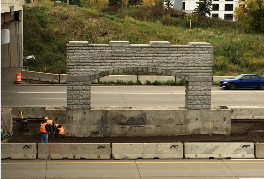
Crews completed the center bridge pier over I-494 in fall 2019. Abutment work is resuming in January 2020.
