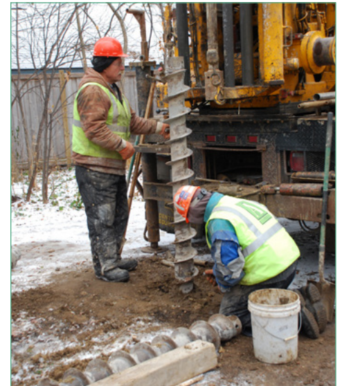
Above: Crews installed additional piezometers in the Kenilworth corridor to monitor ground water levels before LRT construction.
