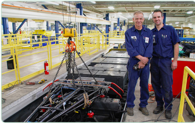
Technicians service the electrical components on the roof of a light rail vehicle at the METRO Blue Line operations and maintenance facility.
