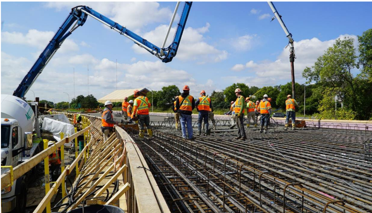
Crews are using a pump truck to place concrete for the Nine Mile Creek Bridge deck.
