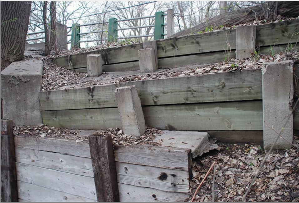
Figure 77. Terraced timber cribbing located at the northeast corner of Bridge No. 6, facing west
