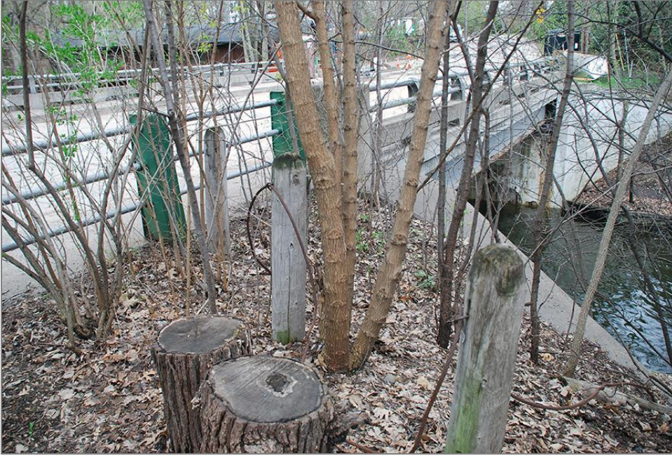
Figure 84. Guardrail on the west side of Burnham Road, north of Bridge No. 6, facing southeast
