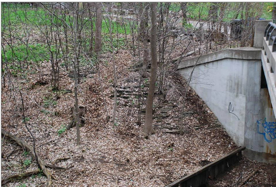
Figure 76. Stone retaining wall located on the northwest corner of Bridge No. 6, facing northeast
