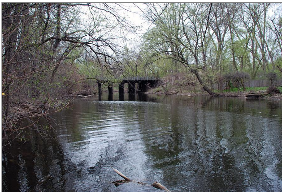
Figure 41. Area between the bridges, with Bridge No. 5 in the distance, facing southeast
