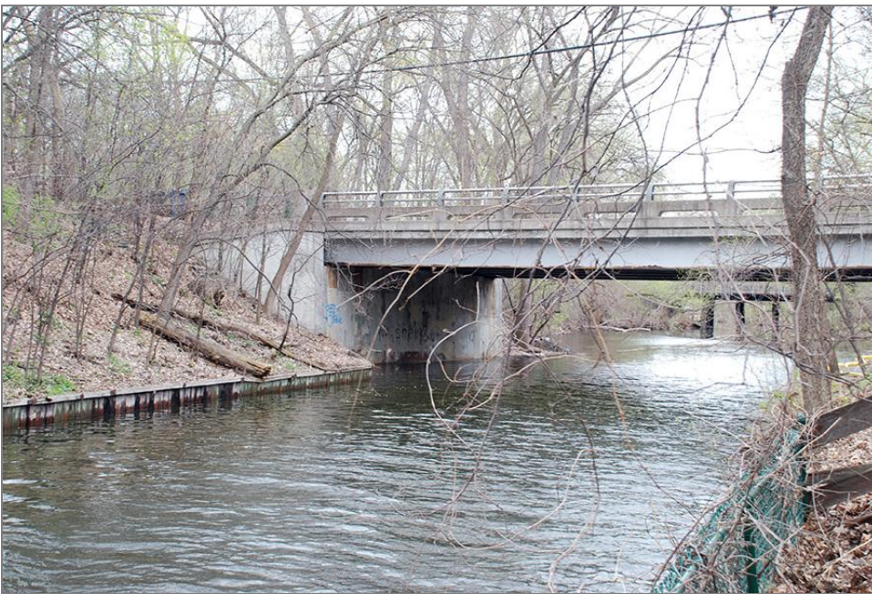
Figure 46. Channel from south shore with Bridge No. 6 in the mid-ground, facing northeast
