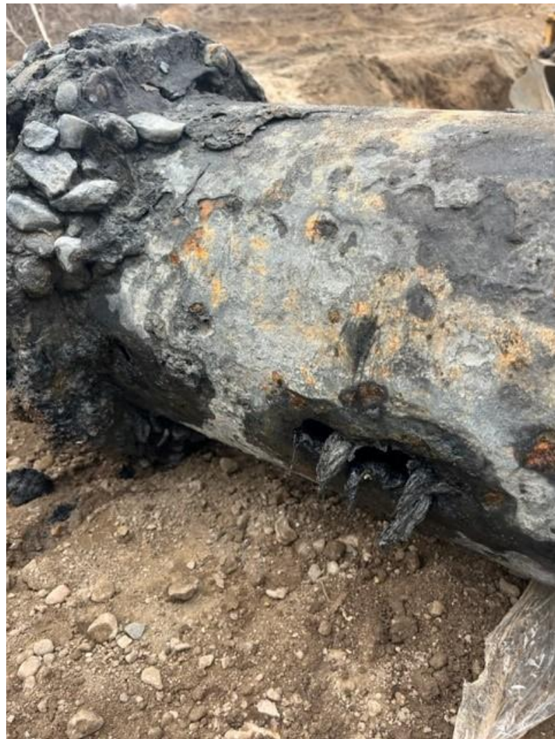
Deteriorated Siphon Pipe - Break
