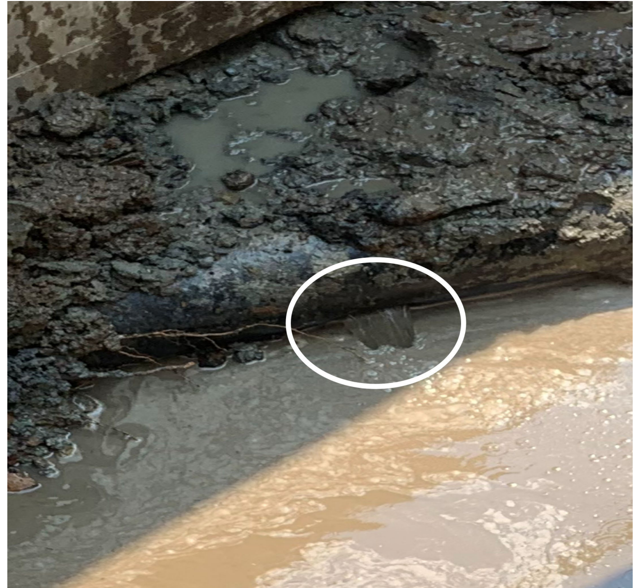
Hole in Pipe
