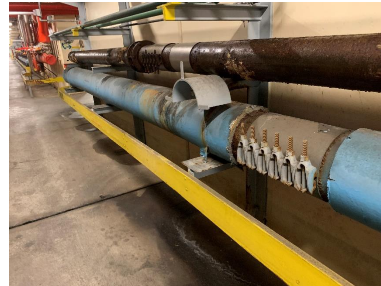
Photo of old steel service water piping showing multiple repairs
