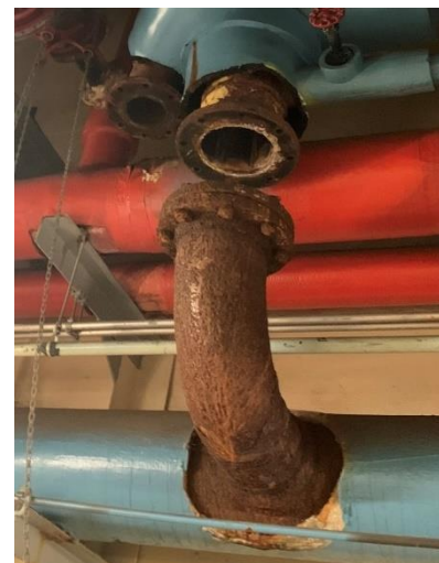
Pipe corrosion on steel service water piping that was covered in insulation.
