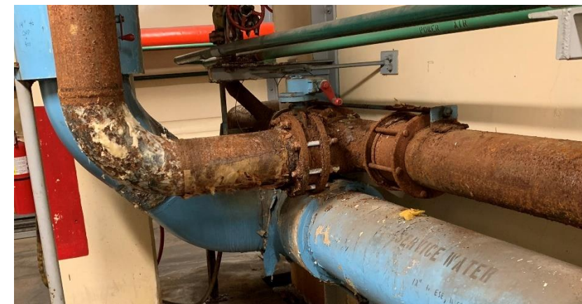
Photo of old corroded steel service water piping and valve
