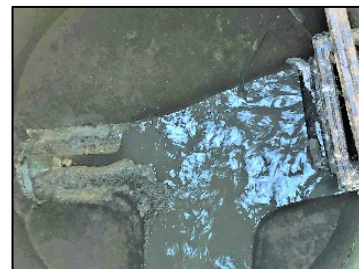
FOG buildup disrupting flow in a local sewer pipe
