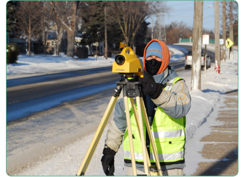
Jeremy Honga of Sambatek does survey work on the Blue Line Extension LRT Project along Broadway Avenue in Robbinsdale
