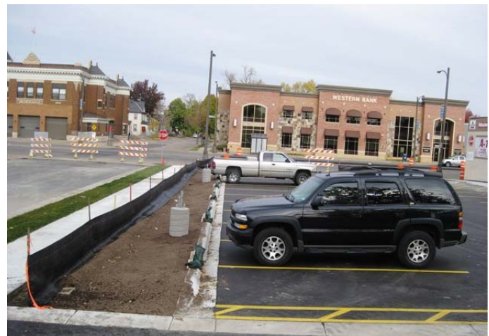
Parking lot improvements near completion at the SE corner of St. Albans and University
