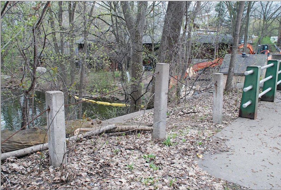
Figure 82. Guardrail on the east side of Burnham Road, north of Bridge No. 6, facing southeast
