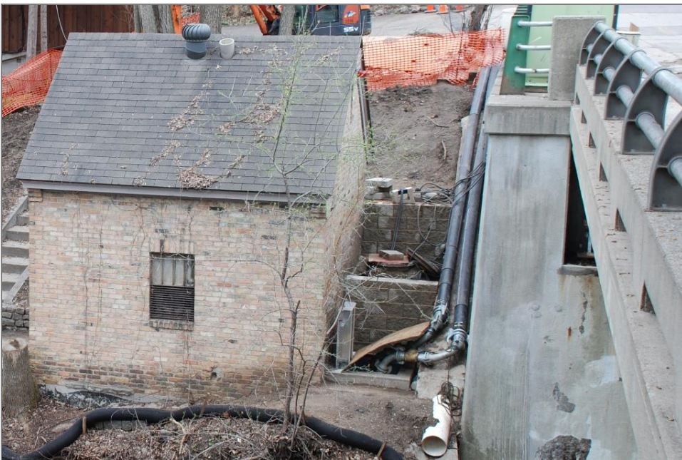
Figure 74. Concrete block retaining wall between the pump house and Bridge No. 5, facing south
