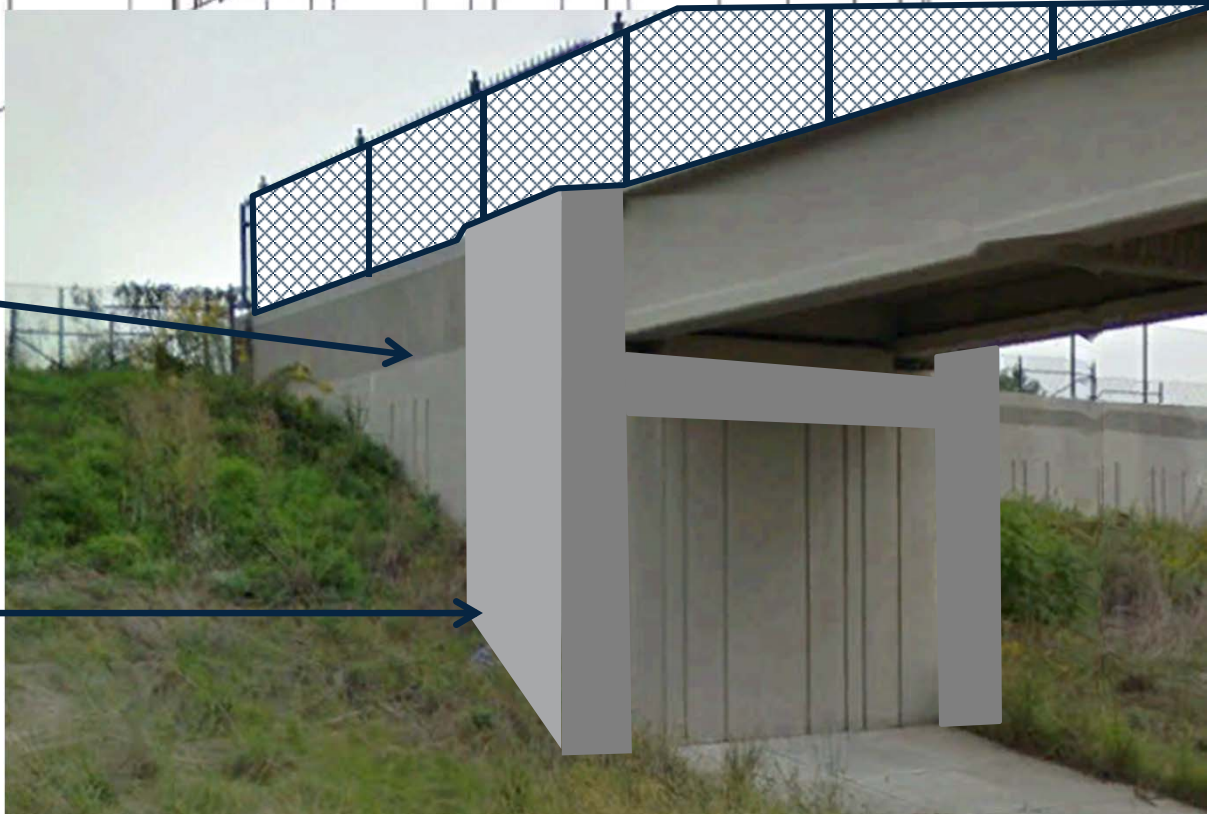
Example of smaller scale bridge abutment with 212 treatment suitable for LRT bridge abutment and wing walls.
